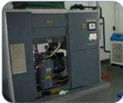
Spare parts not standardized, quality too poor
